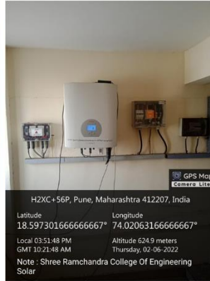
Wheeling To The Grid: Solar Plant
