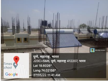
Solar Water Heaters:
